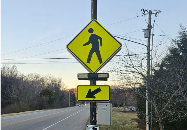
Figure 21. Rectangular Rapid Flashing Beacon (RRFB)
