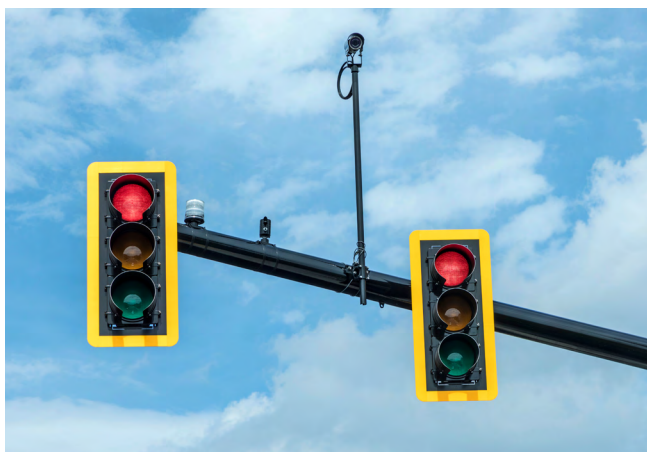
Figure 16. Signal Head on Mast Arm
