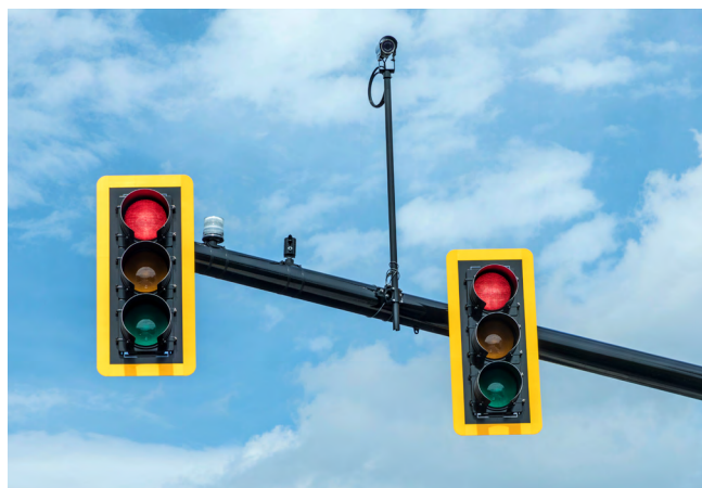
Figure 16. Signal Head on Mast Arm
